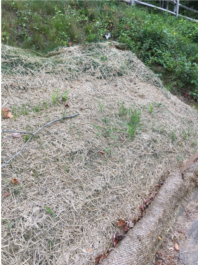
Attempt to remediate erosion by planting more lawn grass, photo Sept. 17, 2020
